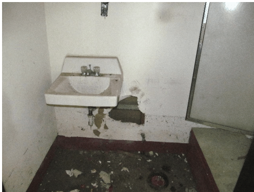
12. Restroom in front store/office area, again illustrating the building's dilapidated condition.
