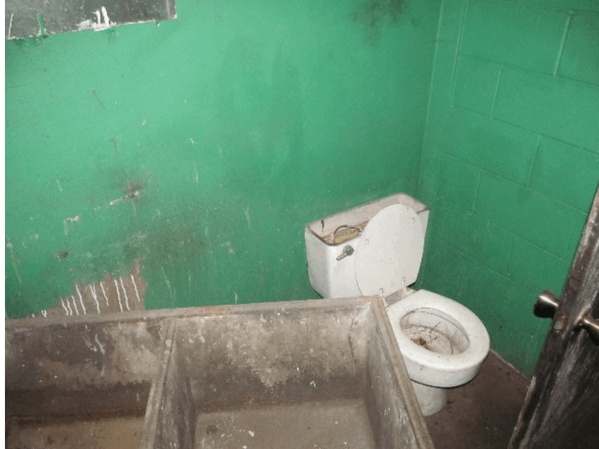
11. Typical restroom in shop area showing heavy wear and tear.
