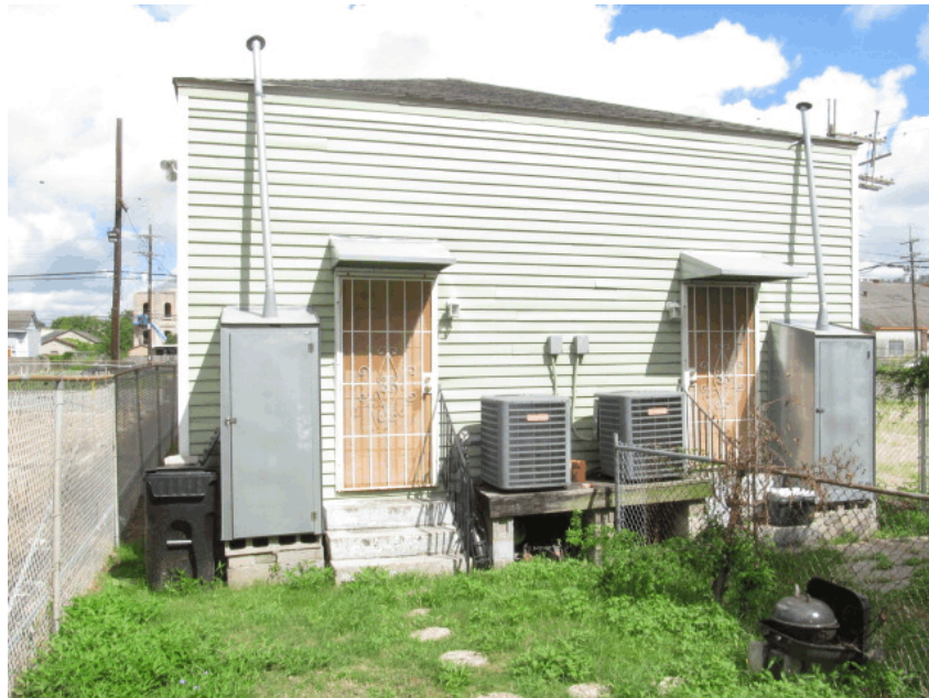
2. Rear view of property as seen from the southeastern corner of the lot.
