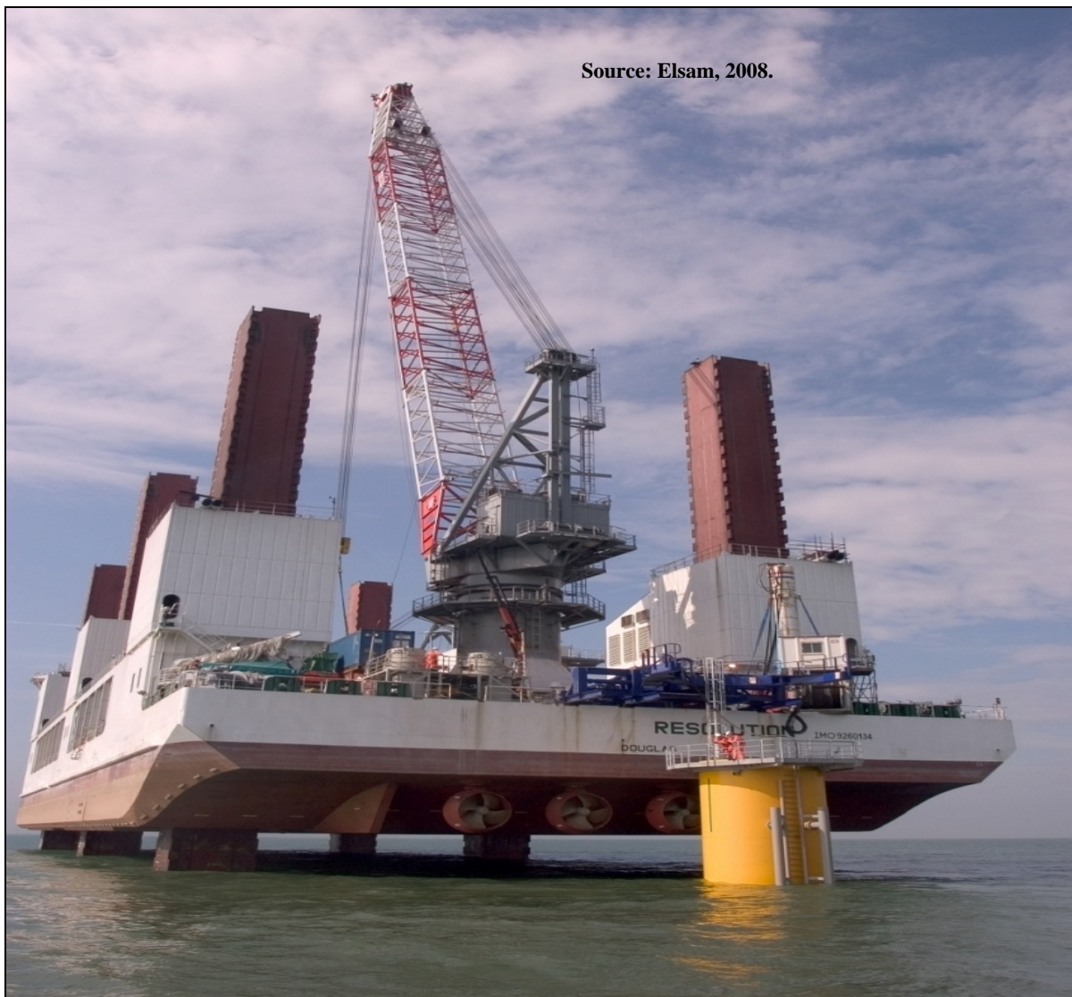
Figure G.12. Monopile after Installation by Jack-Up Barge Resolution at Kentish Flats.
