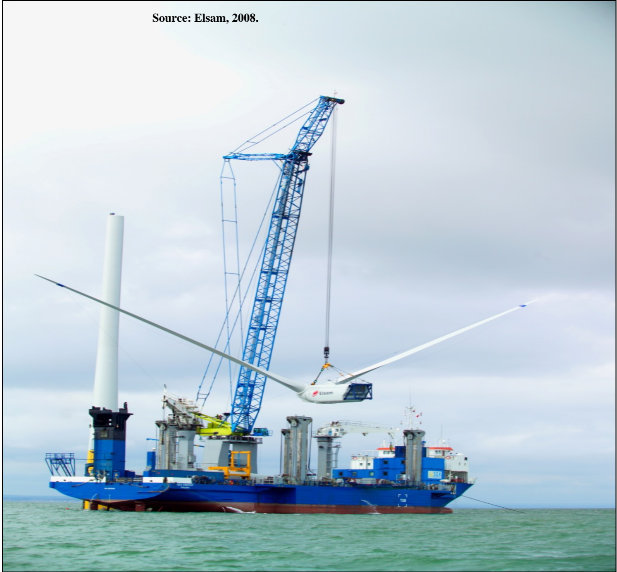
Figure G.13. Nacelle and Blades Being Lifted In Bunny Ear Configuration at Kentish Flats.
