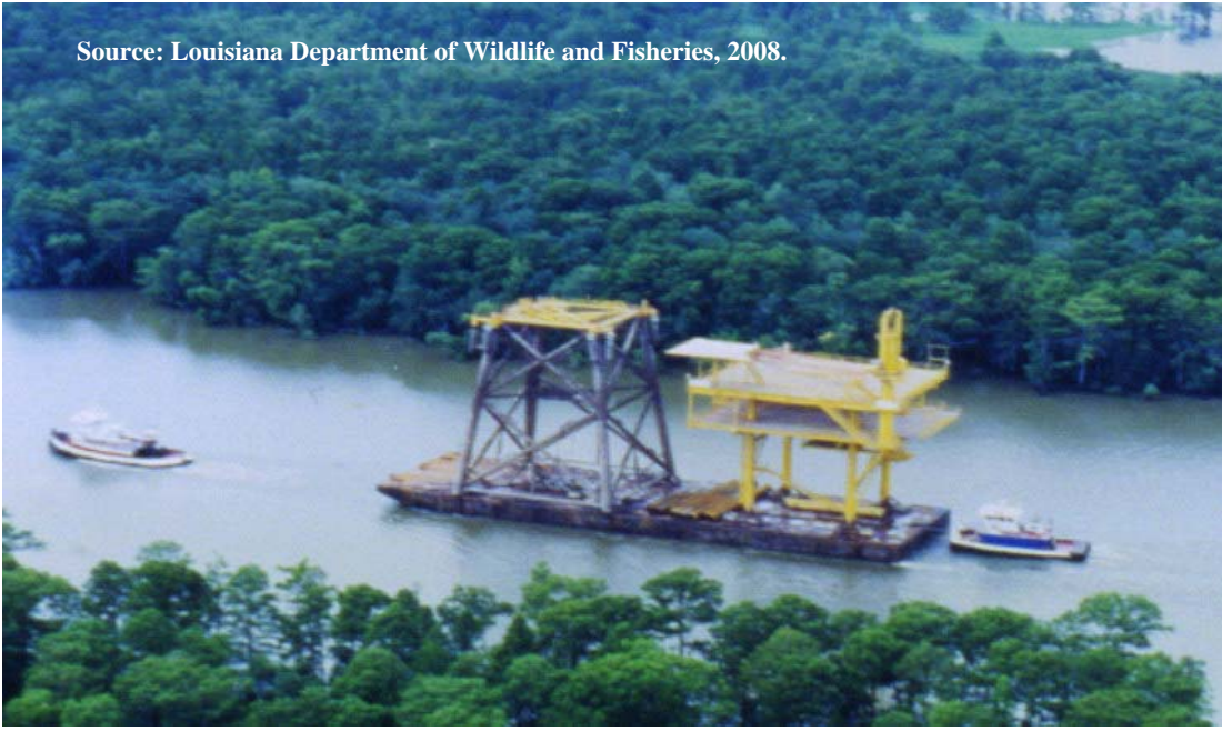
Figure A.14. Jacket and Deck Transported to Shore or Artificial Reef Site.
